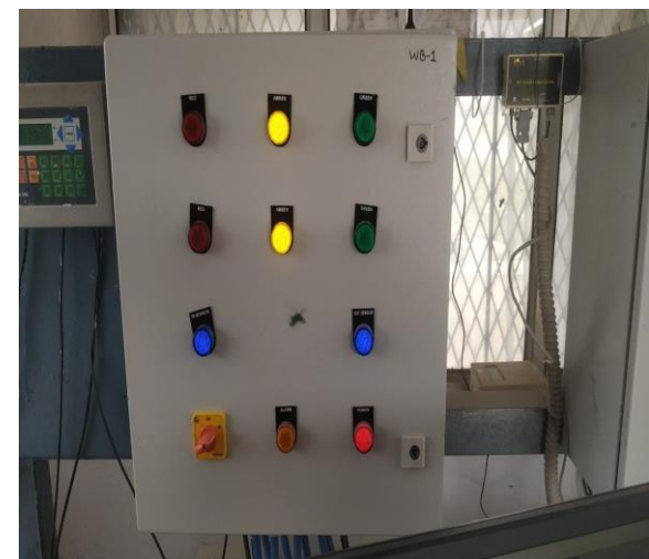
Weigh bridge control panel
